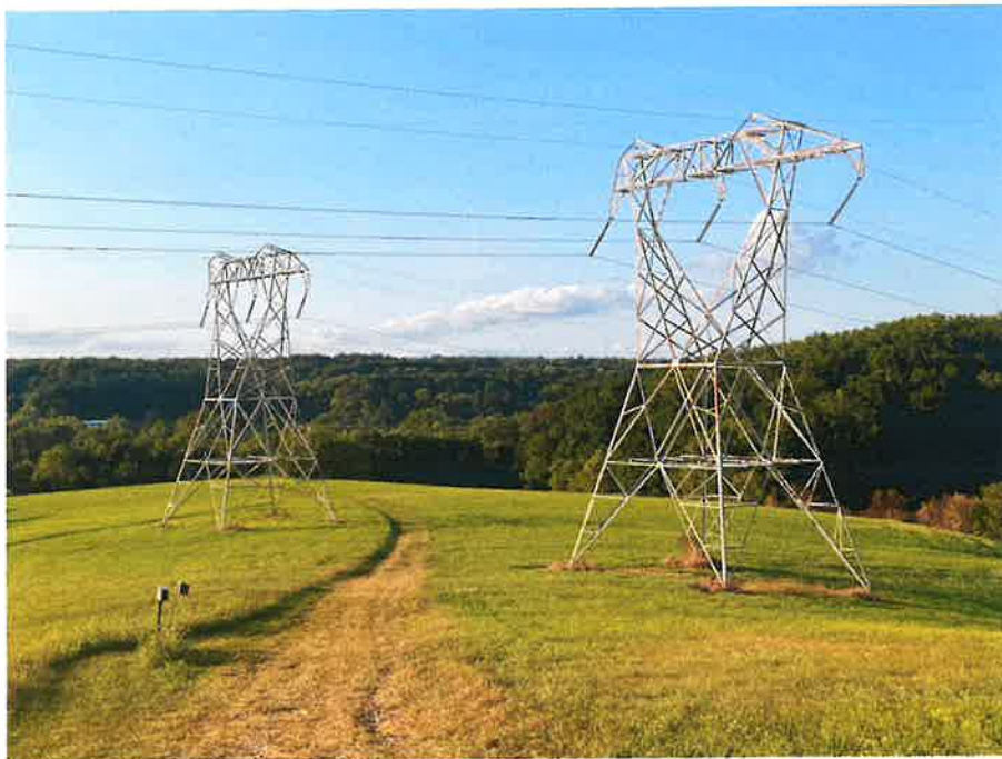
Power lines run across the ChesLen Nature Preserve in Chester County, Pa. (Peter Hall/Capital-Star)
